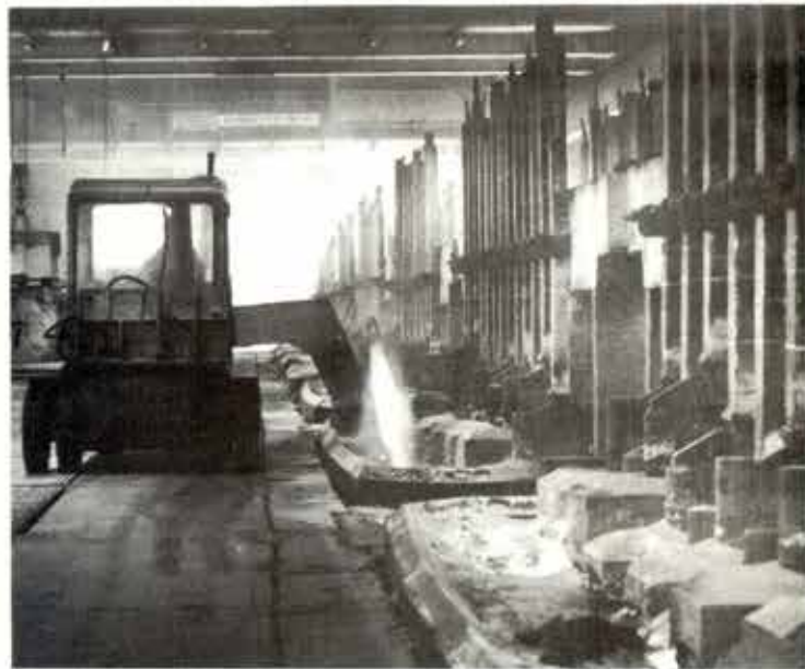
If the first tests prove successful, crustbreakers could be a thing of the past in potrooms one to four.
