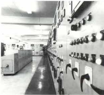
Power to the Potrooms ceased completely for over three hours.
