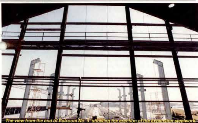
The view from the end of Potroom No. 5 showing the erection of the expansion steelwork.
